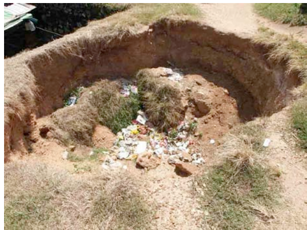
At the Flag Bastion, a hole of 3 meter in diameter is blown in the mud section behind the rampart wall. This is caused by the huge pressure being build up in the sewer system by the tsunami.
