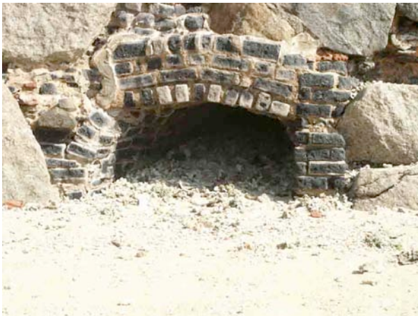
Sewer drain on the outside of the ramparts. One of the two sewer drains is more or less blocked. The other sewer drain washed clean again.
